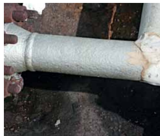
Corrosion Under Insulation
