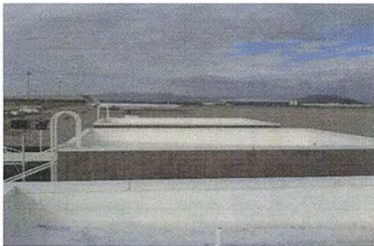
Rental Car Wash roof Before Pressure Wash
