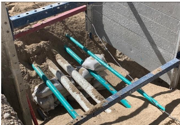
Backfilling of SPI Coatings system for below grade glycol water piping for freeze protection.
