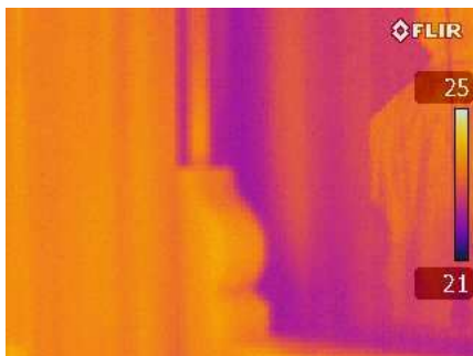
Fig (g): heat leakage around window frame
