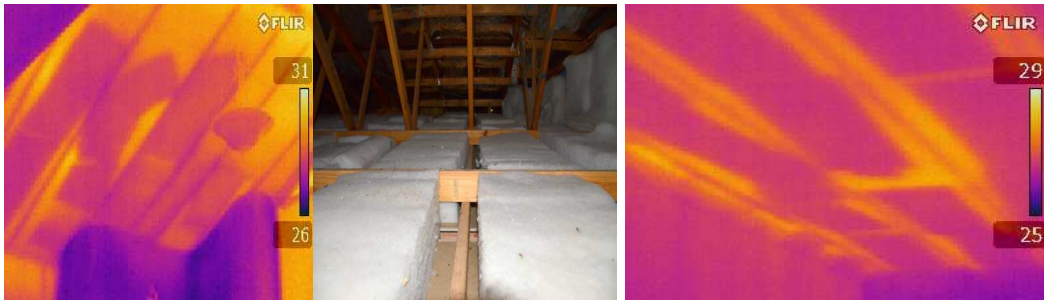
Figure 5.8: Missing insulation as well as large air gaps around insulation, representing serious breaches of BCA regulations
