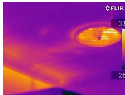
Fig (f): absent draft stopper on vent
