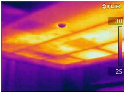
Fig (c): patchy ceiling coverage
